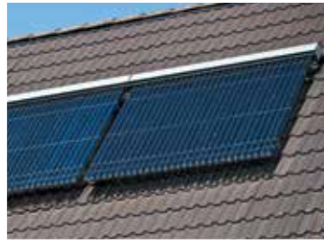
Solar thermal panels 1)
